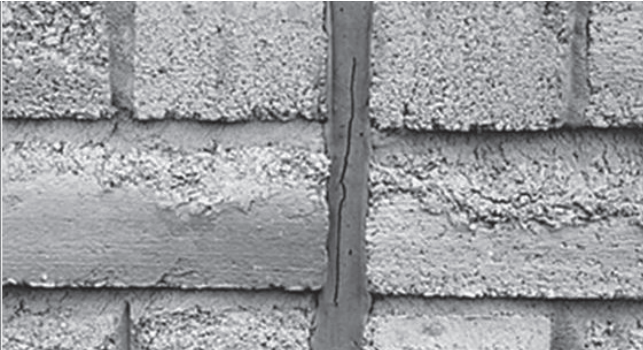
FIGURE 3.7 – SEALANT COHESIVE TEARING
