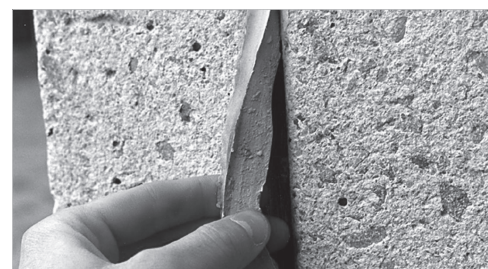
FIGURE 3.6b – SEALANT ADHESIVE BOND LOSS
